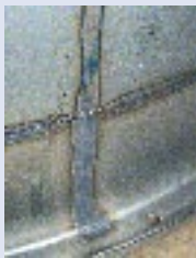
Bluish heat tinting around welds in a 4301 stainless steel tank. If kept un-treated, the risk of pitting corrosion in the bluish zone is significant, and therefore, the heat tinting must be removed. The easiest way to do this is a pickling.
