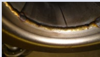
Yellowish weld formed by welding Ti steel (EN 1.4571) with Formier gas. The color doesn't affect corrosion resistance.
